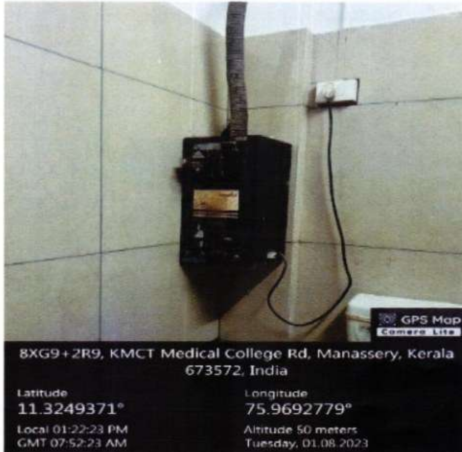
Sanitary Napkin Incinerator
